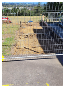
Work has begun on the ramp that will stretch from Kōwhai Āwhina through the bush to the bottom field.
