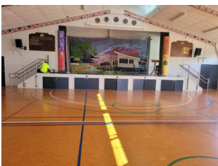
Handrails have been positioned on the stairs leading to both sides of the stage
