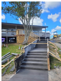
Concrete has been poured for the base of these steps leading from the hall
